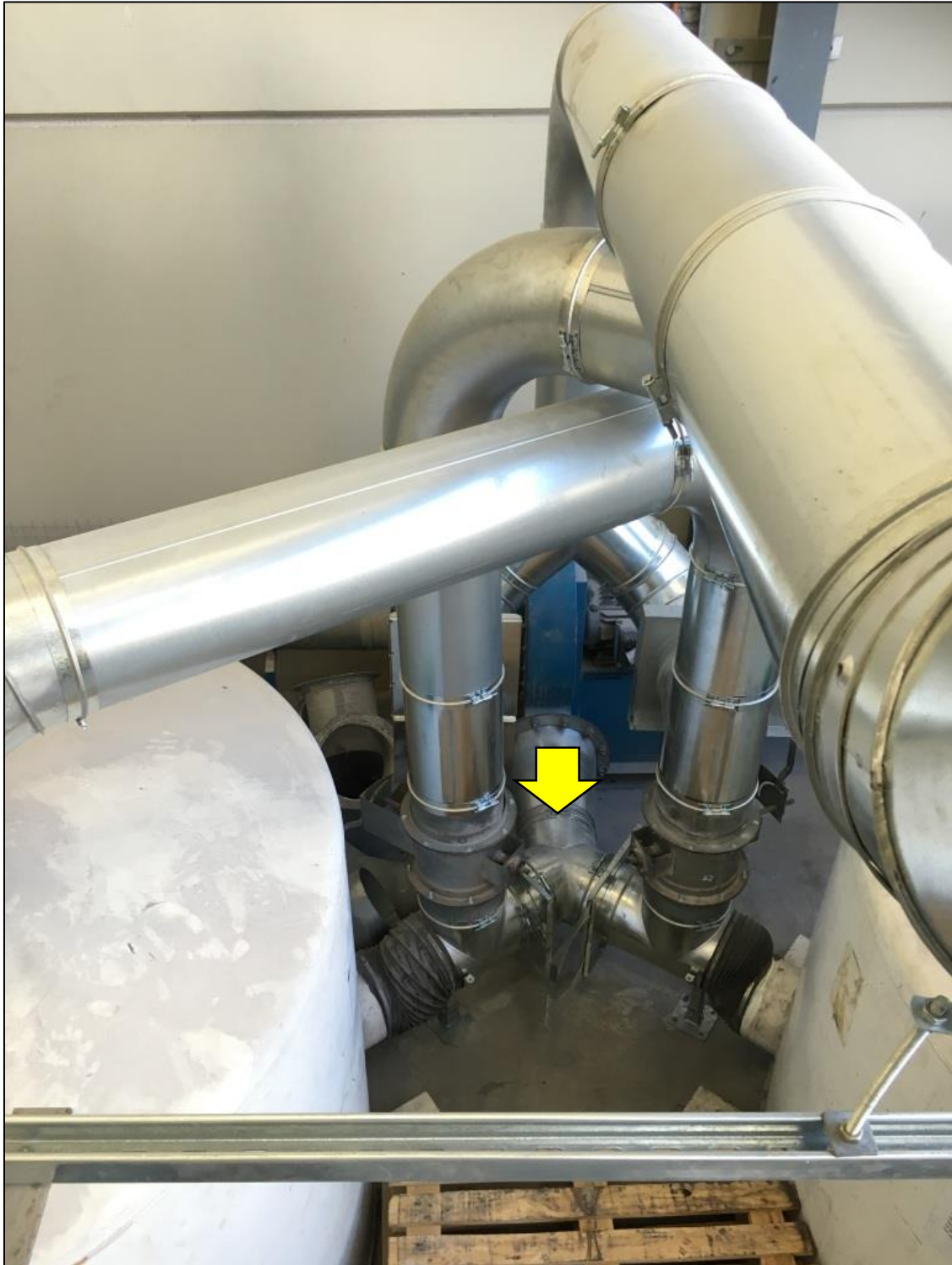
PHOTOGRAPH 2 VARIABLE SPEED FAN EXTRACTING AIR FROM WITHIN PLANT TO SCRUBBER TOWERS IN SERIES
